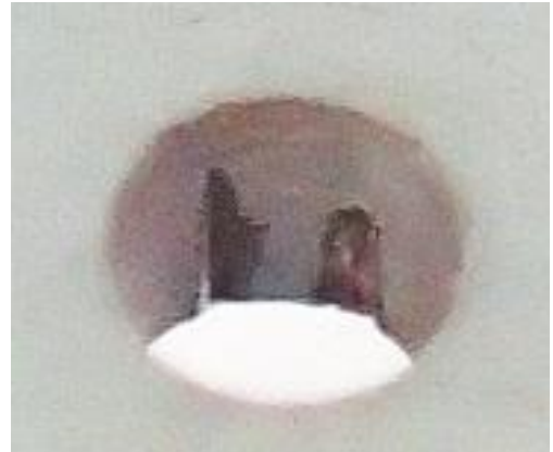
Insertion depth too low
